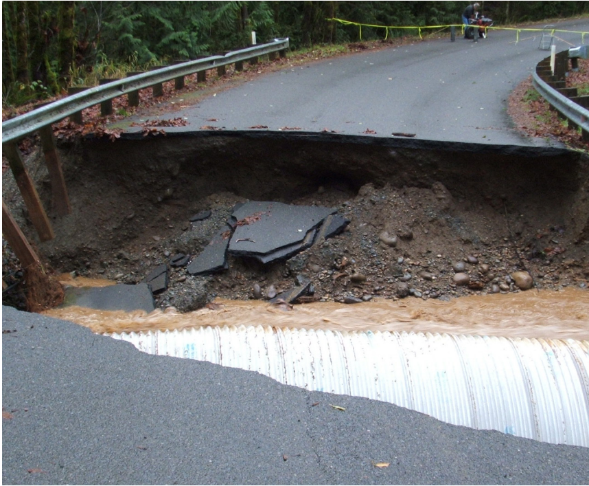
▲ Photo: Flood damage to Cedar Flats Road in Thurston County. [Thurston County Image December 2017]
