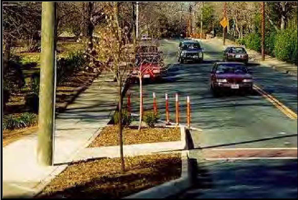
Photo F. View of an actual bump out constructed on busy street.
