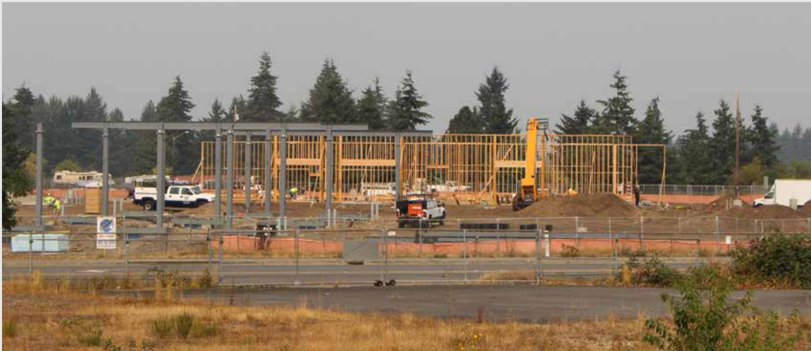
FIG 4: Construction crews built new commercial businesses during summer 2018 near the northwest corner of the US 12 and Elderberry Road/Old Highway 99 intersection, which has become the commercial core of Grand Mound. Such development, which is visible and accessible from I-5, is consistent with the 1996 Grand Mound Subarea Plan's objectives.
