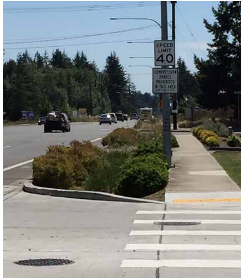
Figure 24: A recently built sidewalk on Old Highway 99, just south of US 12, features a swale ditch planted with shrubs. Such low-impact development helps capture and filter stormwater runoff from surrounding road and sidewalk.
