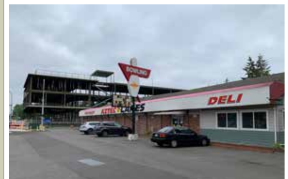
Intercity Transit's new administrative building rises next to the Aztec Lanes Bowling Alley, which was built in 1945.
